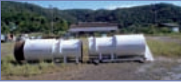
Two-stage fan at Sao Bento mine, installed by Cogmacoustic
